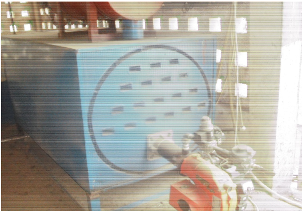
LPG fired heat generator
