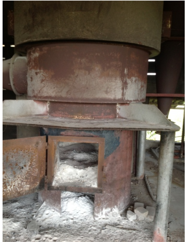
HEAT GENERATION UNIT
