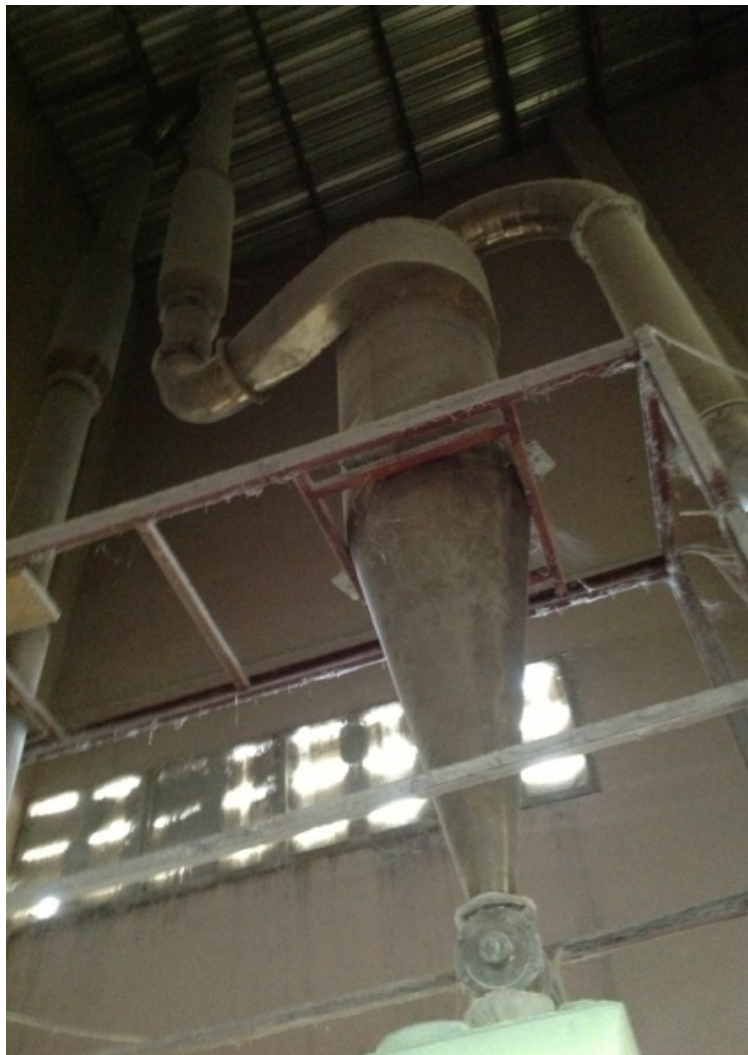
Cyclone of the Flash Dryer at Caltech Ltd.
